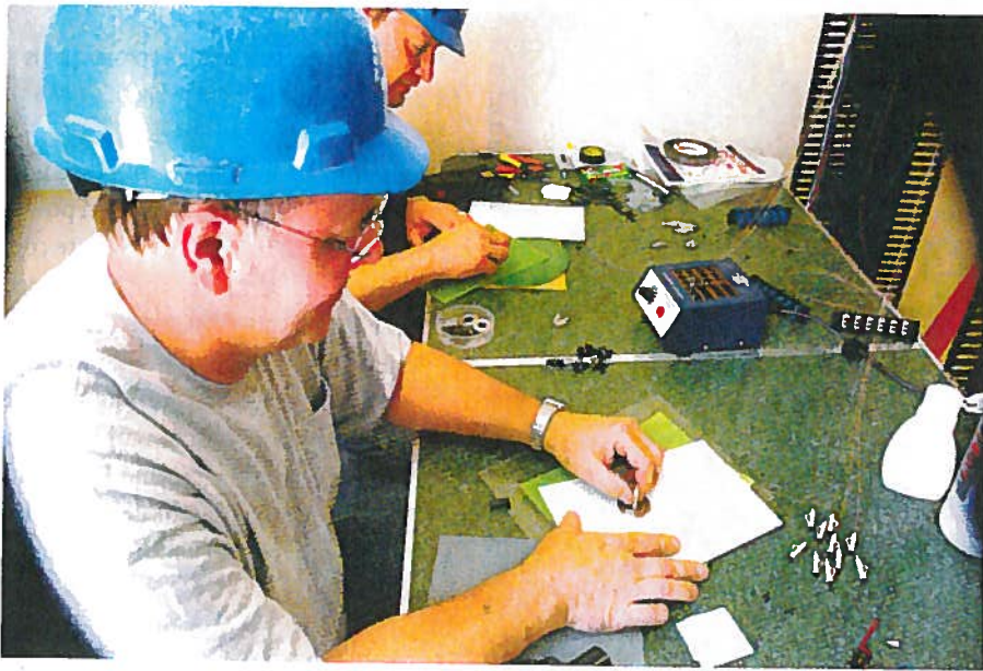
Bruce Campbell and Rich Weirs of Westmoreland Electric Co. polish singlemode and multimode fibers after termination.
