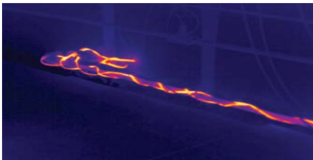
Figure 4 Thermography can even be used for applications such as troubleshooting a heating wire on an outdoor water line, which cannot be allowed to freeze in cold weather.
