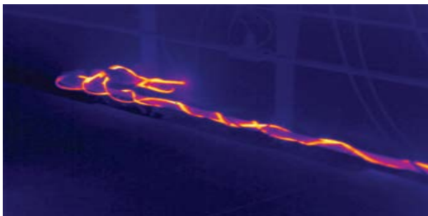
Figure 4 Thermography can even be used for applications such as troubleshooting a heating wire on an outdoor water line, which cannot be allowed to freeze in cold weather.
